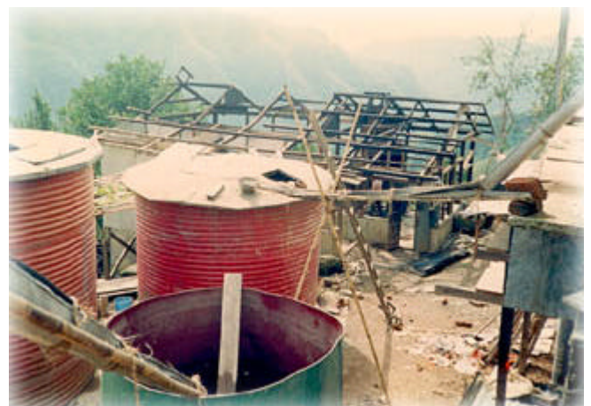
"This snap is of our old kitchen which was blown off by cyclone. Whole roof was gone. This was taken during the repair works. The tanks that you see will give you an idea how we store roof water in rainy"
